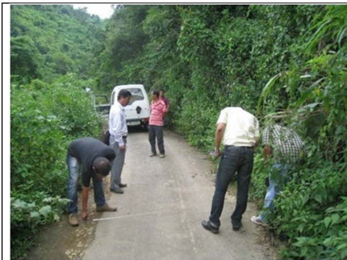
Imphal East: Construction of Road from Luwangsangbam Jn. To Kameng (MN0420) Deficiency in carriageway width i.e. 2.7 m from ch. 3.20 km to 4.70 km
