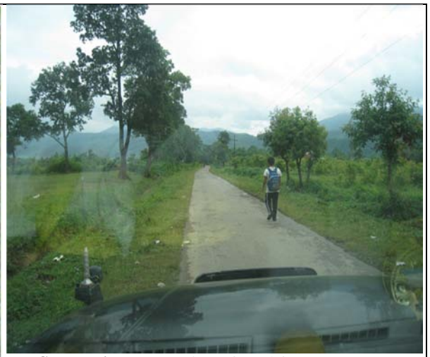
Senapati: Construction of road from NH39 to Saikotjang Part II (7.77 to 15.37 Km): Recording of excavation in plain areas
