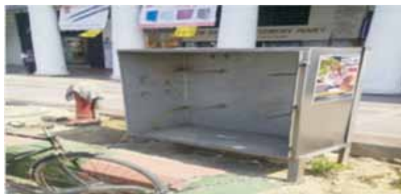
Empty and damaged Fire Hydrant Box
