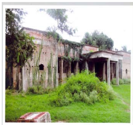
Abandoned work of Civil Surgeon office and office-cum-residence (38F2/07-08 of Darbhanga Division)
