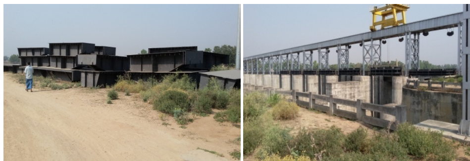
Photograph of Punpun Barrage showing incomplete erection work of the barrage
