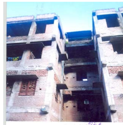
Abandoned 3rd grade staff quarter at PMCH, Patna (9F2/07-08 of Construction Division No.-1, Patna)
