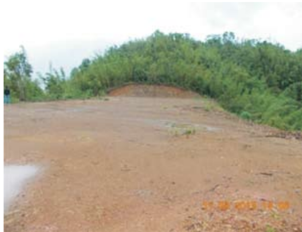
Site preparation for Administrative and Workshop Building at ITI Serchhip at Chhiahtlang Village
