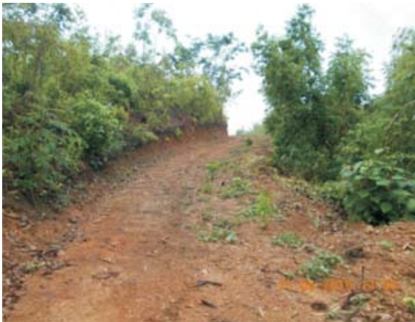
Site preparation for approach road to ITI Serchhip at Chhiahtlang village, Serchhip
