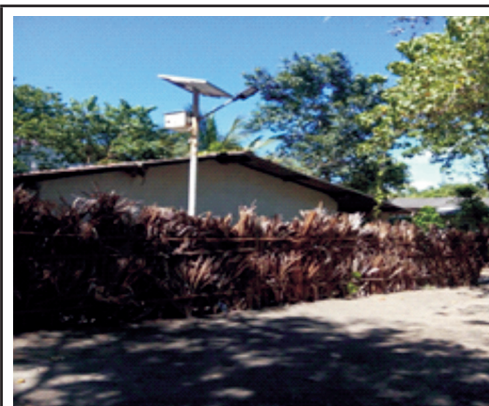
Picture 6 : SPV SLS installed in the residential premises of GP member of Village Dehari, Taluka Umargaon, District Valsad (11.06.2015)
