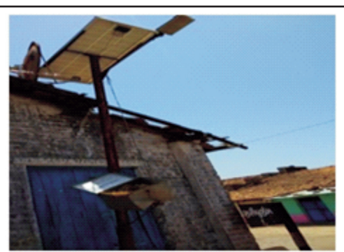
Picture 4 : The SPV SLS of Village Zaribuzarg, Taluka Garbada District Dahod was non-functional within six months from the date of installation (18.05.2015)
