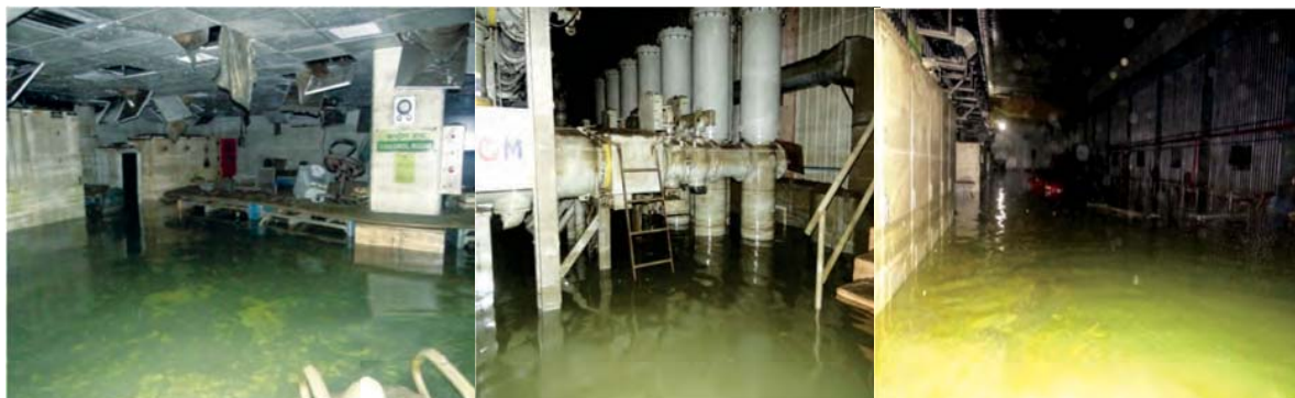
Flooding in Dhauliganga Power House
