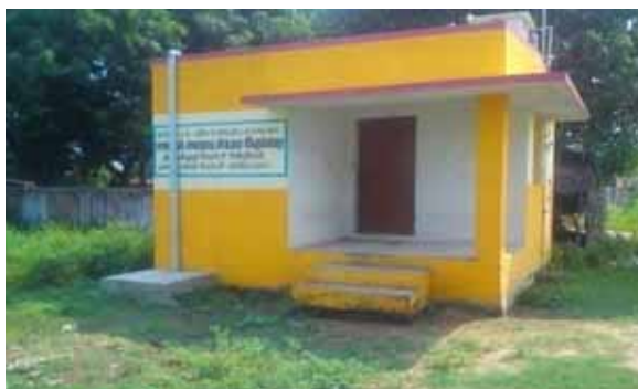
Photo 15: KCS was not handed over by the contractor for 2 years as a result the constructed building was not used (PUMS, Pullarambakkam School)
