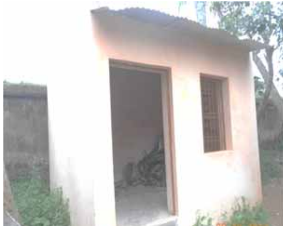
Photo 17: Cooking of MDM was not done in the newly constructed kitchen shed due to small size(10'X9')
