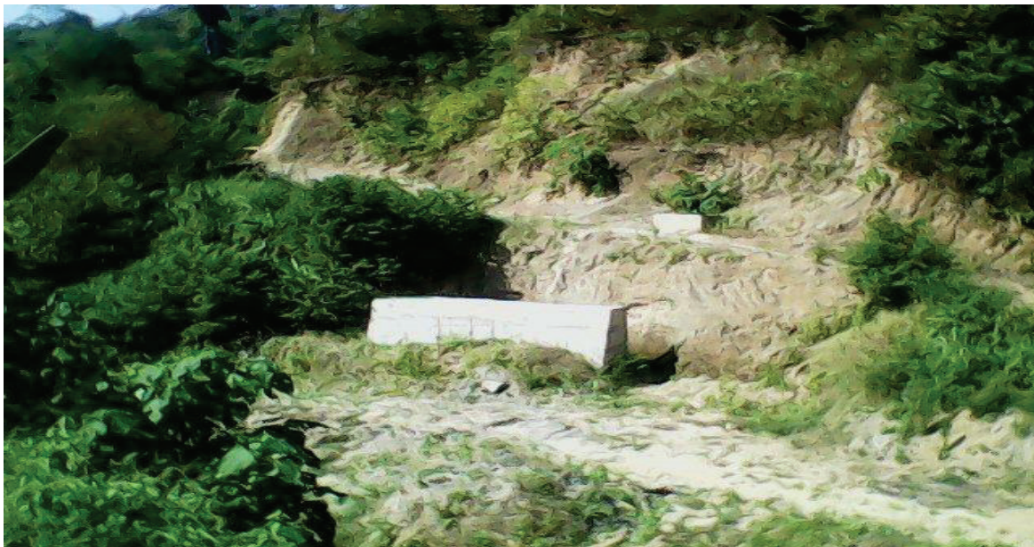
Picture 4.1: Incomplete Bridge and unconnected road at Sukhovi in Nagaland
