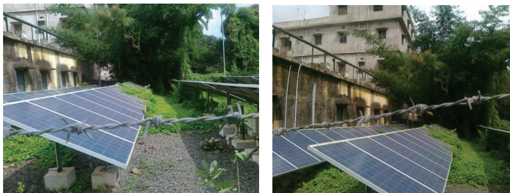
(Solar plates of off-grid Solar Power Plant at Jasidih, Deoghar covered with grass)
