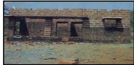
Photo of incomplete Mahavir Community Hall at Tadaki Hill side, Khordha
