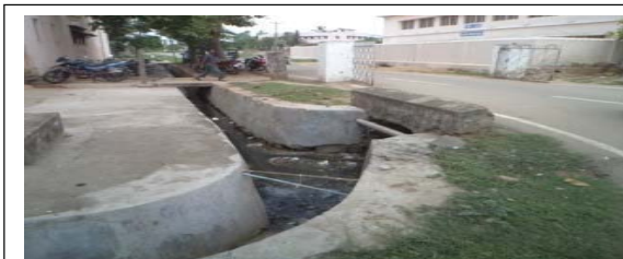
Waste water directly discharged to drain of Berhampur City
