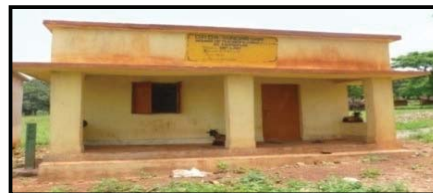
Photograph of Community Centre at Kamanda in Kulta GP of Koiria Block lying idle without being handed over
