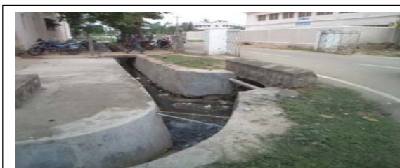
Waste water directly discharged to drain of Berhampur City
