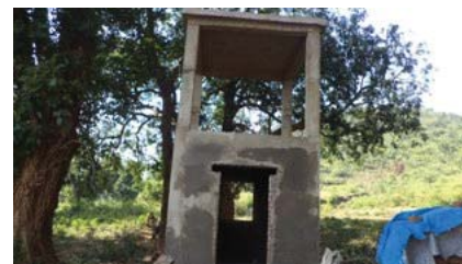
Incomplete bore well at Bariguda, Gadagada VDC, Bissam Cuttack Block
