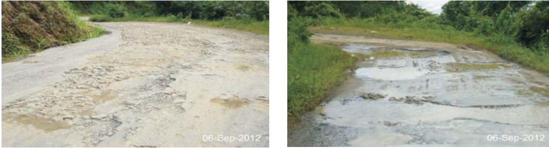
Stone filling and Water logging in Pot Holes in Lunglei – Tlabung Road (9.00 - 39.00 kmp)
