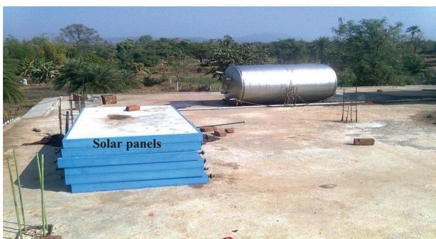
Solar water heater system lying uninstalled in KGBV, Dahanu
