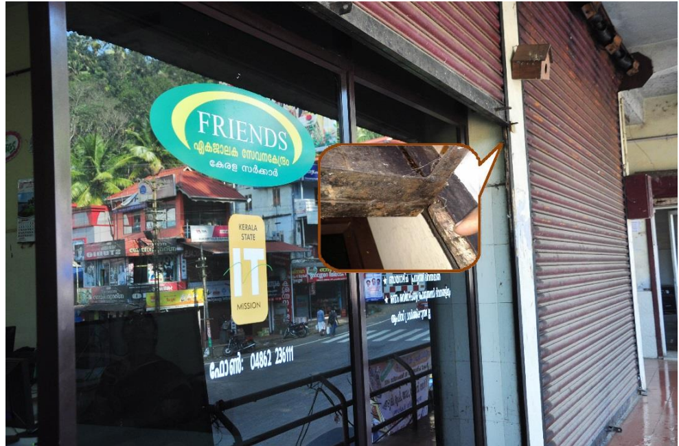
Picture depicts view of Idukki Centre, where the steel shutter cannot be closed. The shutter channel is blocked with wooden logs to prevent collapsing of the damaged steel shutter. Inset picture displays a wooden log used as blockade.
