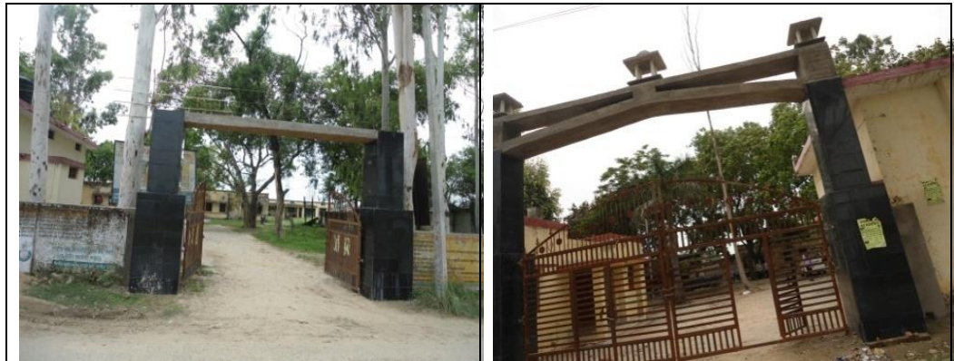
Construction of two gates in the campus of BDO office of KP Mardah, Ghazipur.
