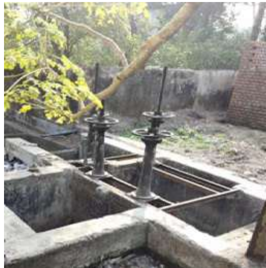
Exhibit 6.10: Pump house of the partially functional STP of the Jiaganj-Azmiganj Municipality
