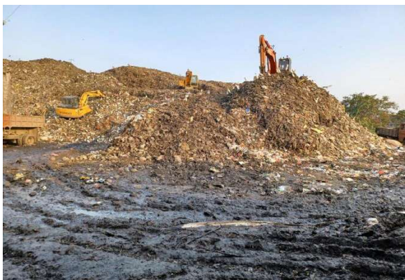
Exhibit 6.3: Heaps of garbage at the Ramchandrapur dumping Ground, in the Panihati Municipality
