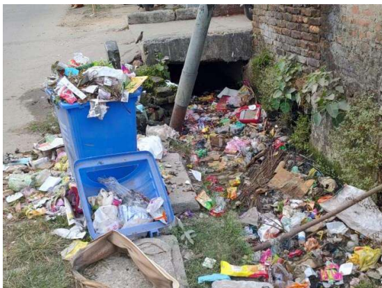
Exhibit 6.7: Clogged drain at Ward no. 07, at the Tufanganj Municipality
