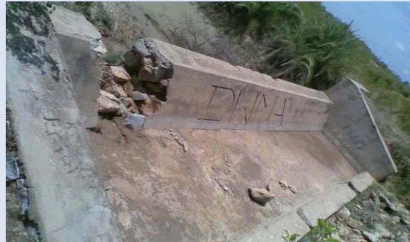
Name of the project: Chalkurthanda Name of the district: Anantapur Non-repaired check dam with toe wall and apron
