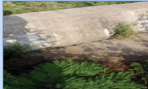
Name of the project: Murlinagar Name of the district: Rangareddy Incomplete check dam – Non construction of apron, etc.
