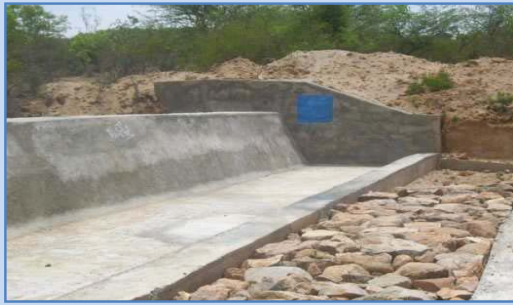
Name of the project: Pulumamidi Name of the district: Rangareddy Incomplete check dam – Non-clearance of excavated soil
