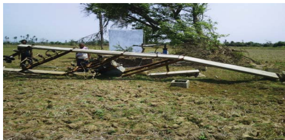
LIP at Agasti Nuagaon-1 village under Chhatrapur Block not restored
