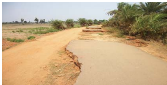
Bipulingi to Gangapur road fully washed and not restored
