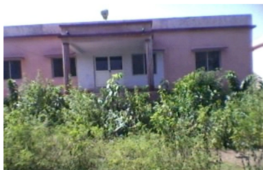
Non-functional CHC building at Boipariguda
