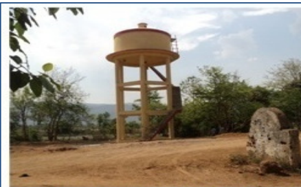
Elevated storage reservoir of RPWS to Makarsala in Kalahandi district without pump house and external electrification works
