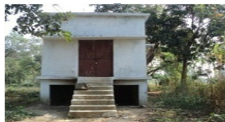
Photograph of RPWS at Janged in Bargarh district which remained non functional due to non completion of electrification works
