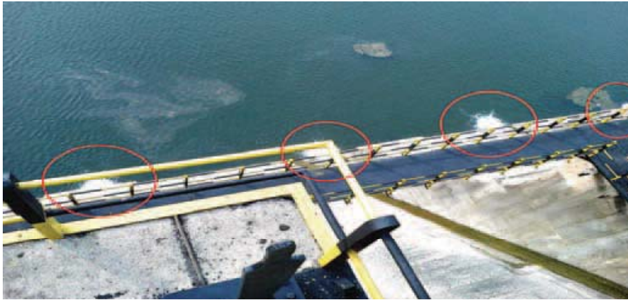
Leakages in Ujjani dam
