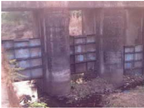
Non-functioning cross regulators at chainage 26/765
