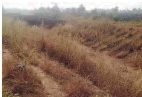
Grass in main canal bed
