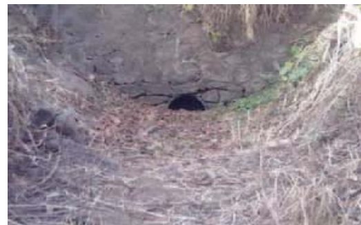
Off taking distributary blocked at chainage 32/985
