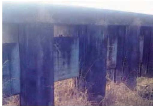
Non-functioning cross regulators at chainage 21/500
