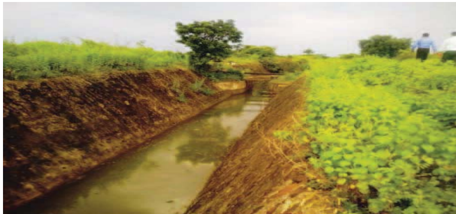
Vegetation growth and water leakage from head regulator in canal, Sirsinala Project, Nagpur
