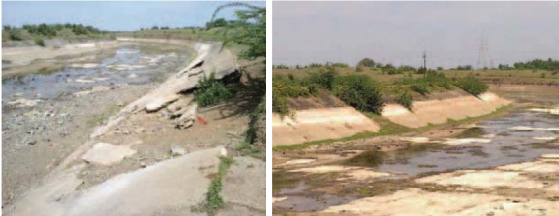
Damaged lining of Ujjani LBC
