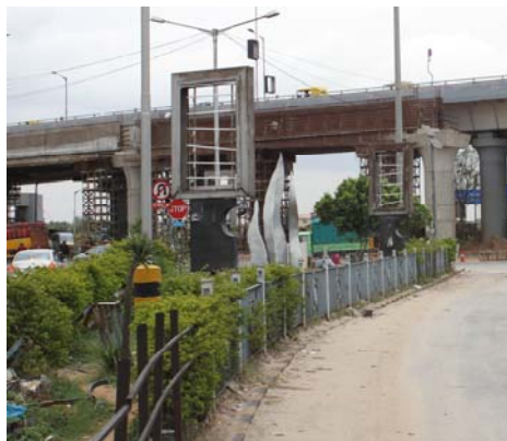
Damaged advertisement boards at Hebbal flyover
