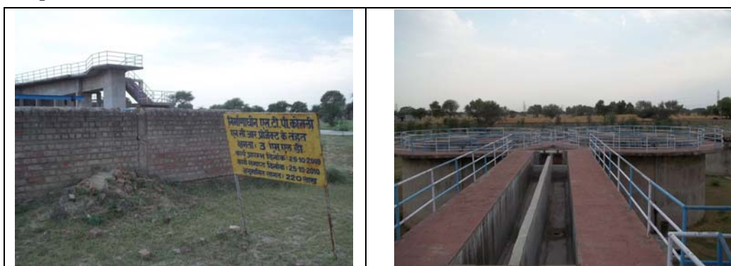
Unutilized three MLD STP at Kosli due to incomplete main sewer line joining STP and non-availability of land for outlet disposal channel carrying treated domestic wastewater (2 April 2013)
