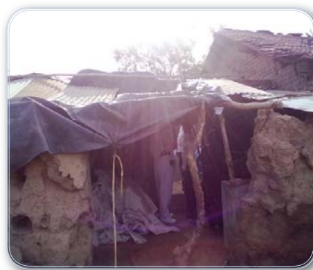
Picture 2 IAY houses of Parmar Jasiben Jinabhai, Village Moraj, Taluka Tarapur, District Anand (29.05.2013)
