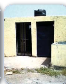
Picture 4 Toilet in Chavaj PS, Bharuch without water connection (29.05.2013)
