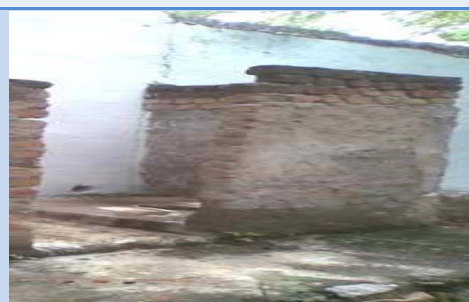
Gram Panchayat: Thummalacheruvu Mandal: Ghattu District: Mahbubnagar IHHL without door, roof and devoid of water
