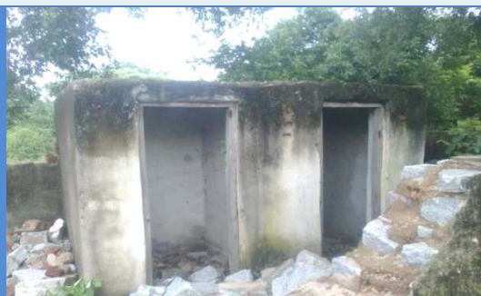
School: Mandal Praja Parishad School Gram Panchayat: Gudimunkanpally Mandal: Damaragidda District: Mahbubnagar Toilets not in use due to dilapidated condition
