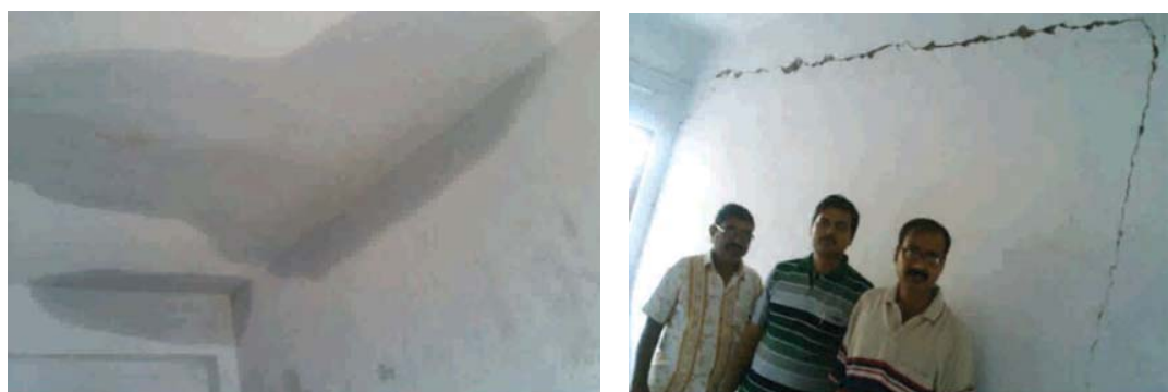
Seepage (left) and crack (right) on the ceiling and walls of hostel at Kotshila
