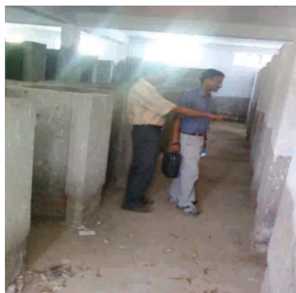
Ground floor where bathrooms and toilets were not fitted with doors and other bathroom fittings. Floors were also not complete.
