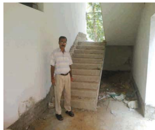
Incomplete flooring and stairs without handrail.
