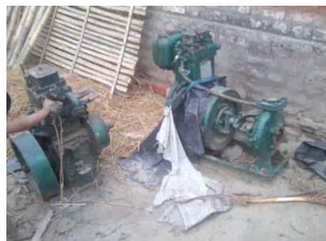
Diesel Generator set to be installed in RLI lying uninstalled on the road side in Asrafpur-III, Malda.
