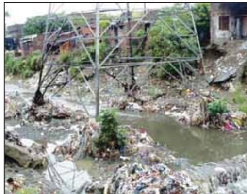
File photo of position of tower with damaged foundation at Bindal River, Dehradun
