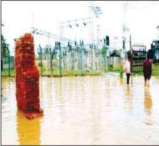
File photo of Switch yard of 132 KV SS at Laksar during flood
