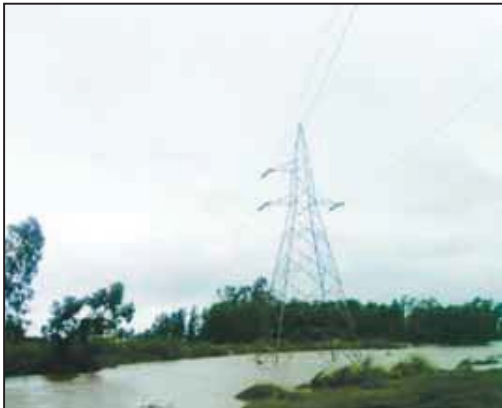
File photo of Feeder of 132 KV SS at Kashipur during flood
