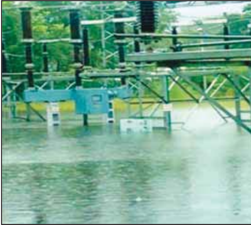
File photo of Switch yard of 132KV SS Bhopatwala Haridwar during flood
