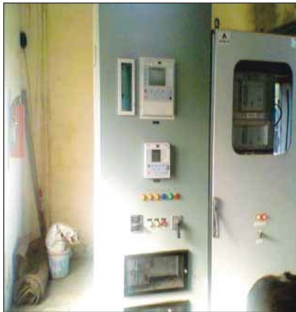
Un-connected Panel of the bus coupler at 132KV SS, Kashipur
