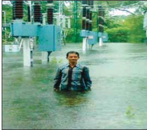
File photo of 132KV SS Bhopatwala Haridwar during flood
