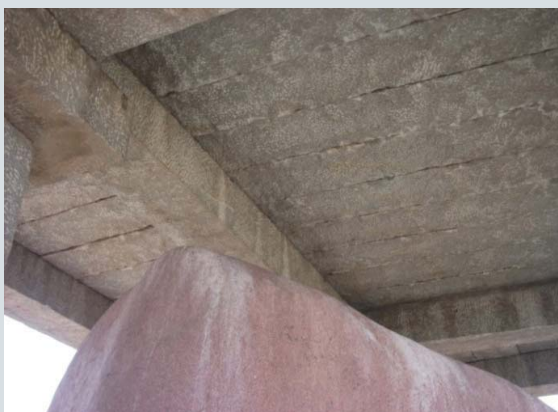
Stains due to water seepage at Ashokan Rock Edict at Nittur, Dharwad
