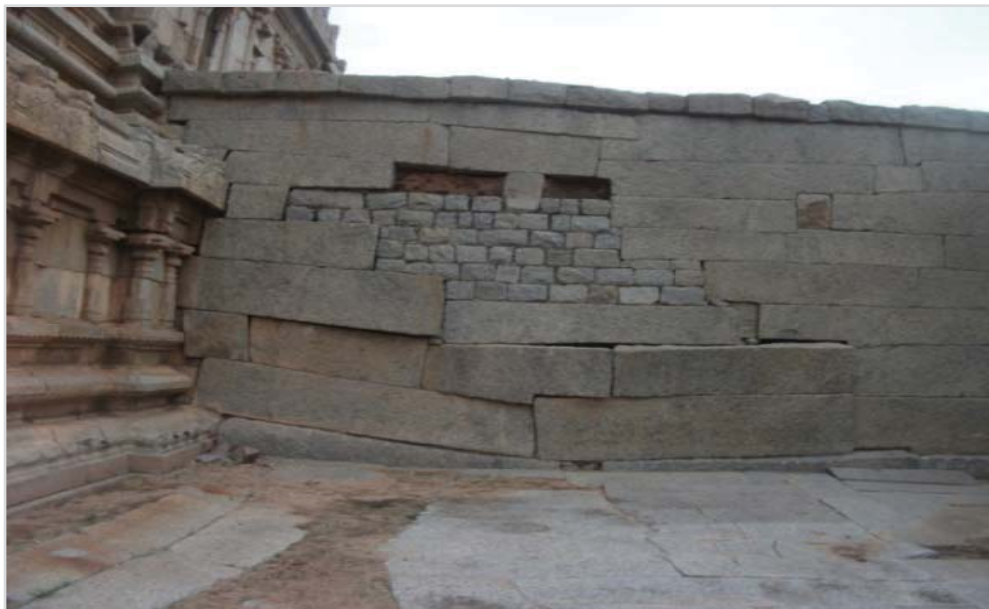
Cracks in Krishna Temple, Hampi, Bengaluru Circle
