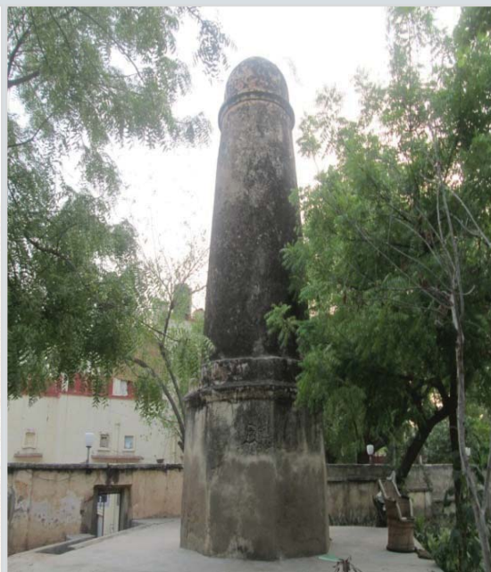
Kos Minar at Jaipur – Ajmer Road, Ajmer encroached by the residence of SP, Ajmer
