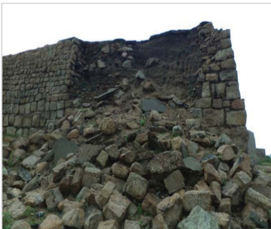
Chinnakavandanur, Sangagiri – Fort bastion in a damaged condition
