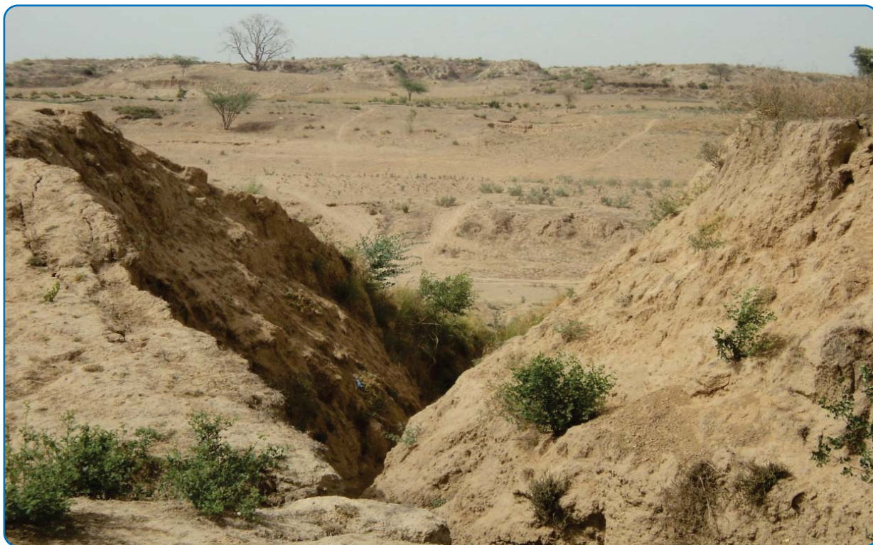
Damaged check dam at Atar Singh ki dhani, GP Bajna block Rajakhera, district Dholpur, Rajasthan
