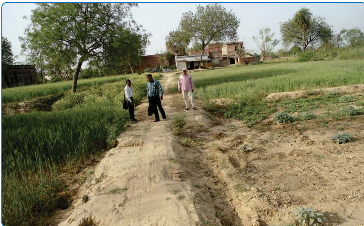
Broken earthen road constructed under MGNREGS, gram panchayat-Khalispur, block Chiraigaon, district Varanasi, Uttar Pradesh
