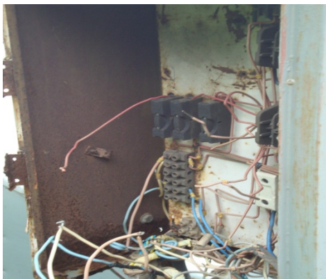
Electrical Panels of the Lock Gate
