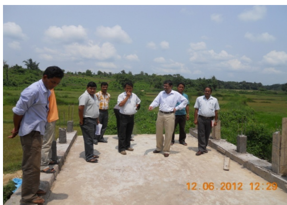
Construction of box culvert near Dasher Ghat SB School at Surendranagar ADC village under Hezamara RD Block
