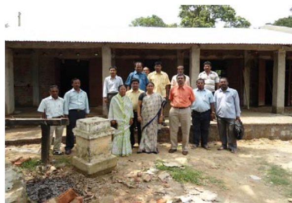
Construction of Rajib Gandhi Seva Kendra at Salghara GP of Matabari RD Block
