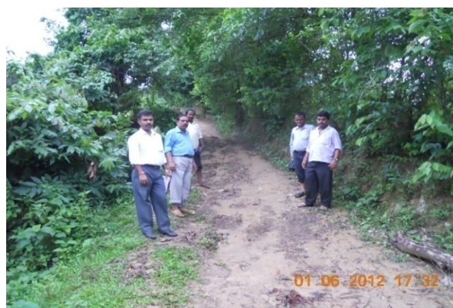
Formation of road from the land of Ranjit Das to Chindrai Para under Paschim Howaibari GP
