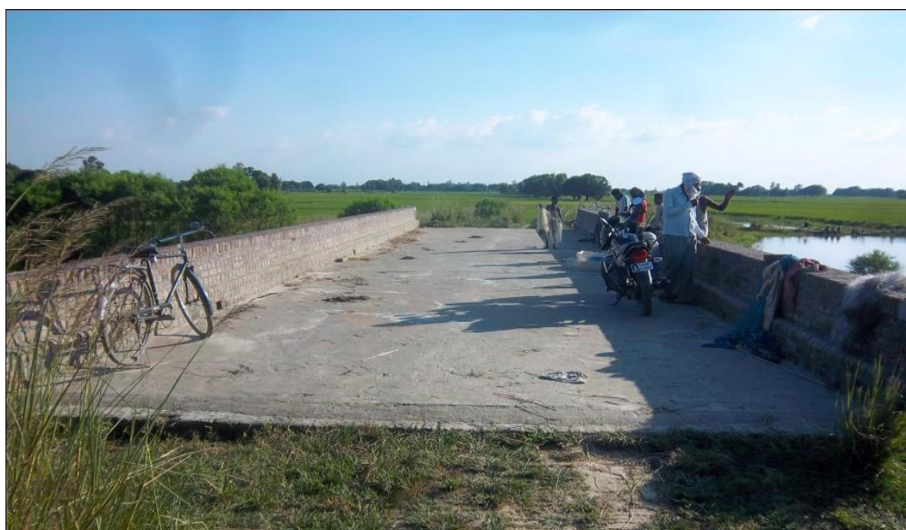
Awabpura Raj Awabpura Rajbhar Basti to Deoria Tal bridge and approach work
