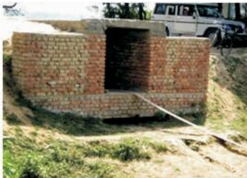
Scheme No.8/10-11 PS-Lakhnaur: Foundation was not constructed
