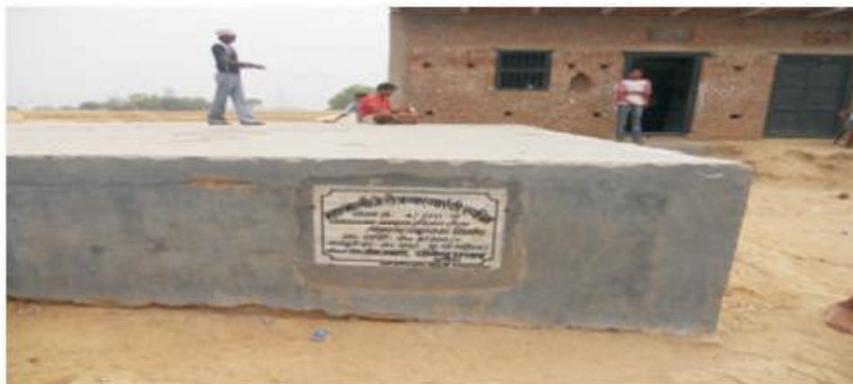
Scheme No.- 4/11-12; GP-Dihara, PS-Obra (Aurangabad) Pucca platform was constructed in violation of MGNREGS guidelines.
