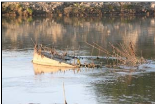
SHIFT AND TILT OF SUBMERGED PIER NO.1 (26/12/2011)
