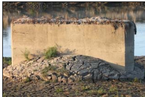
PIER NO. 2 WHERE HEAVY SILTING OCCURRED (26/12/2011)
