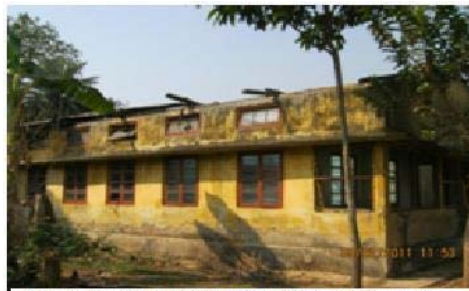
Dilapidated hostel building at RFTI, Amranga (February 2011)
