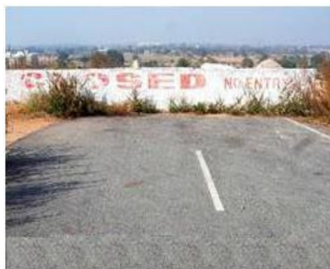
Road closed at verge of the cliff
