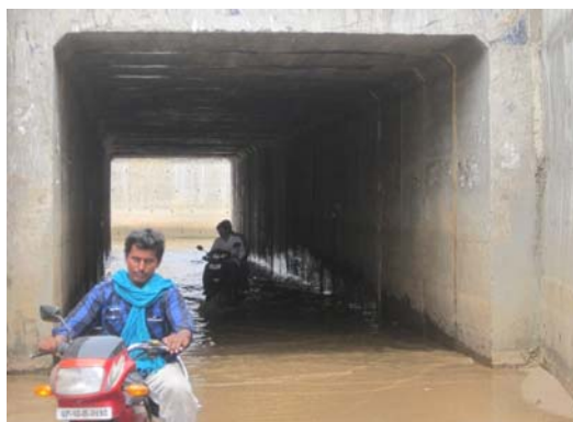
Photograph showing water stagnation resulting in obstruction to traffic at RUB at Puttur Town
