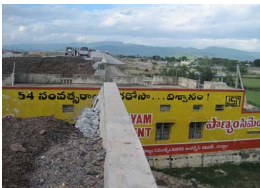
Approach for ROB on SH 30 at Renigunta affected due to land acquisition problem
