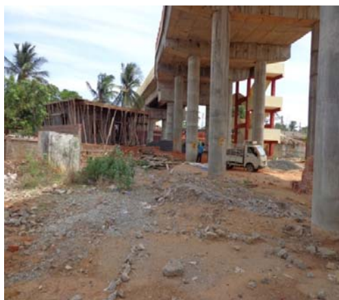
Extra height of bed blocks added by Railways to match height of deck slabs at ROB at Anaparthi
