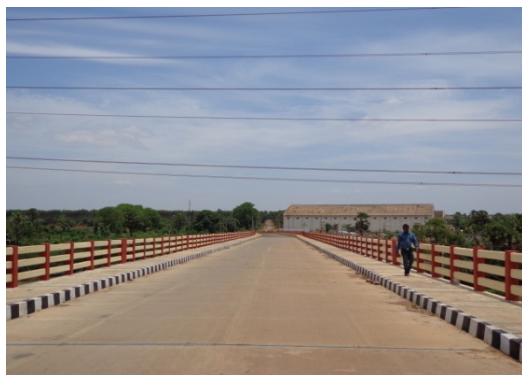
Perilous state of ROB at Bhalabhadrapuram vis-à-vis 220KV and 400KV HT lines
