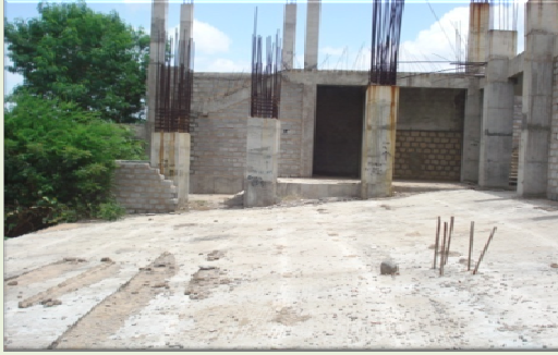
Dismantled RCC slabs and stage beam of Auditorium at JNTU, Anantapur (10 August 2012)
