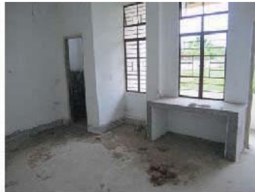
Nagaland- BSUP project, Kohima: DU constructed with single room at Burma Camp- Photo Taken on 08/06/2011
