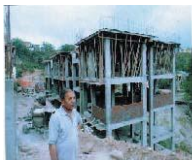
Block Nos. 1 to 6 of IHSDP project in Hamirpur, Himachal Pradesh under construction (18 May 2011)
