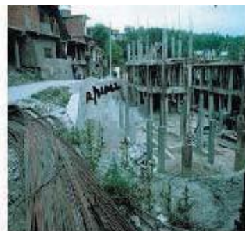
Block Nos. 7 and 8 of IHSDP project in Hamirpur, Himachal Pradesh under construction (18 May 2011)
