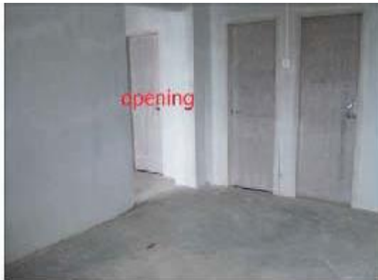
Nagaland- BSUP project, Kohima: Two DUs with opening on the adjoining walls – Photo taken on 03/06/2011
