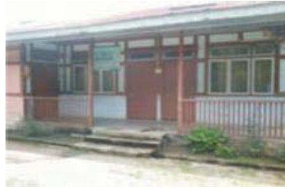
Existing (old) guest house utilised for Community Service Centre (CSC) and Gram Prasasan Kendra
