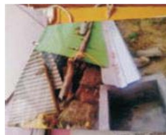
Inferior work of Rain Roof Harvesting
