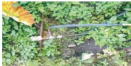
tapping Unauthorised en-route
