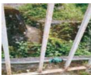
Leakage of water
