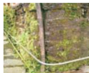
Pipe bent instead of using tee, bend, etc.
