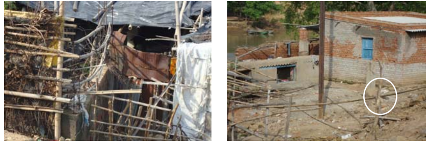
Photographs showing the remaining parts of demolished structure and demolished column of marketing complex
