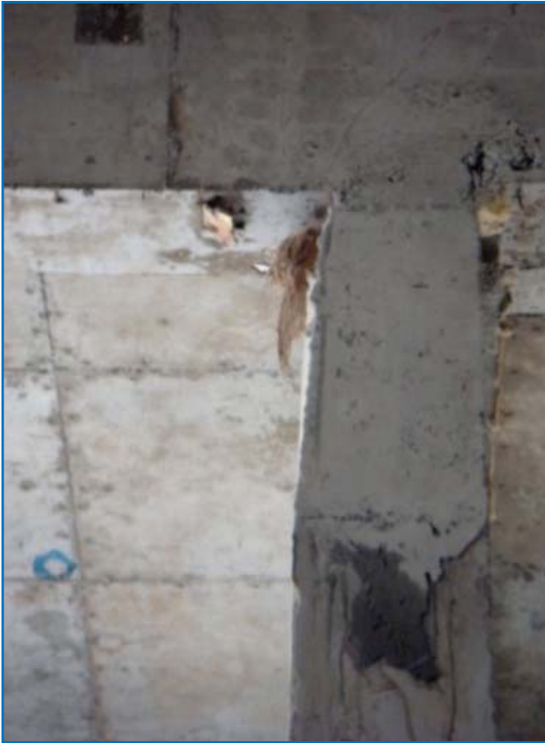
Tapered and Bent up Column in the Basement of Tower-3 (Report No. 3)
