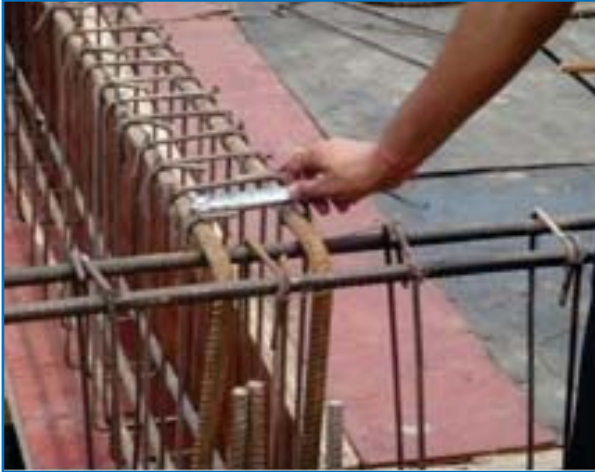
Inadequate hook length and absence of 135° angle reported in CBRI Report No. 2
