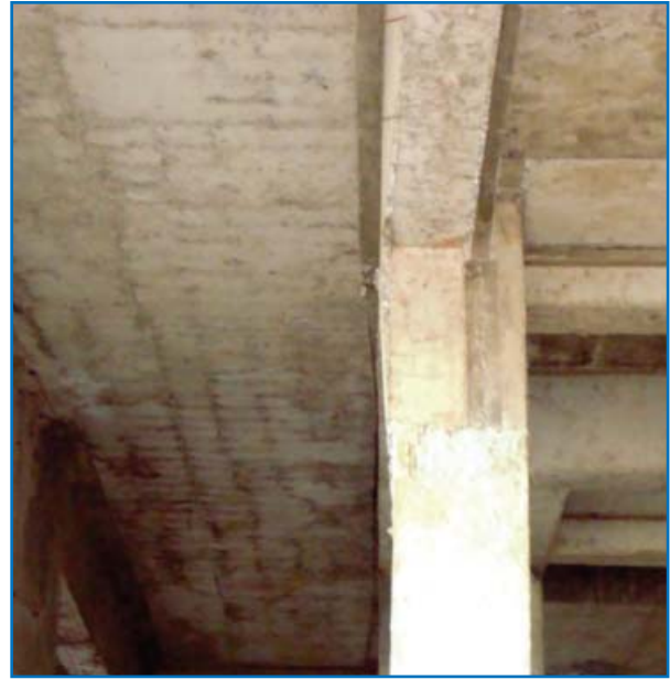
Two in one: Tilt of the column and lack of cover for the reinforcing steel (Tower-34, Upper Basement) Report No. 9
