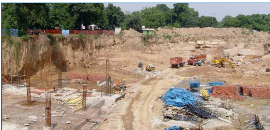
Picture of the construction site at Talkatora Indoor stadium indicating space available for construction activity.
