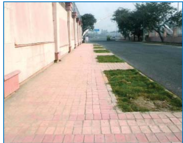
M-30 grade interlocking paver block meant for heavy traffic laid on footpath
