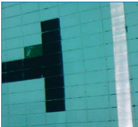
Poor quality of tiling work executed in the pool
