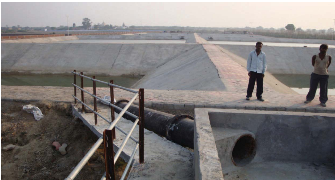
Incomplete STP 2.76 mld (WSP technique) at Mathura
