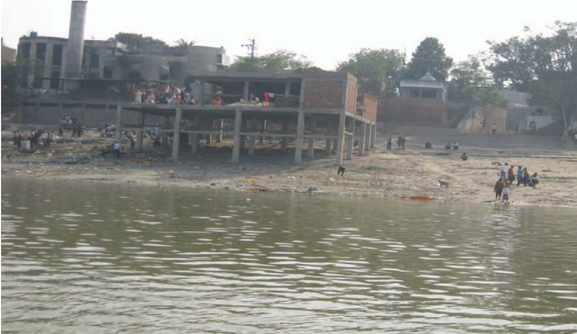
Incomplete RFD at Gulbi ghat, Patna
