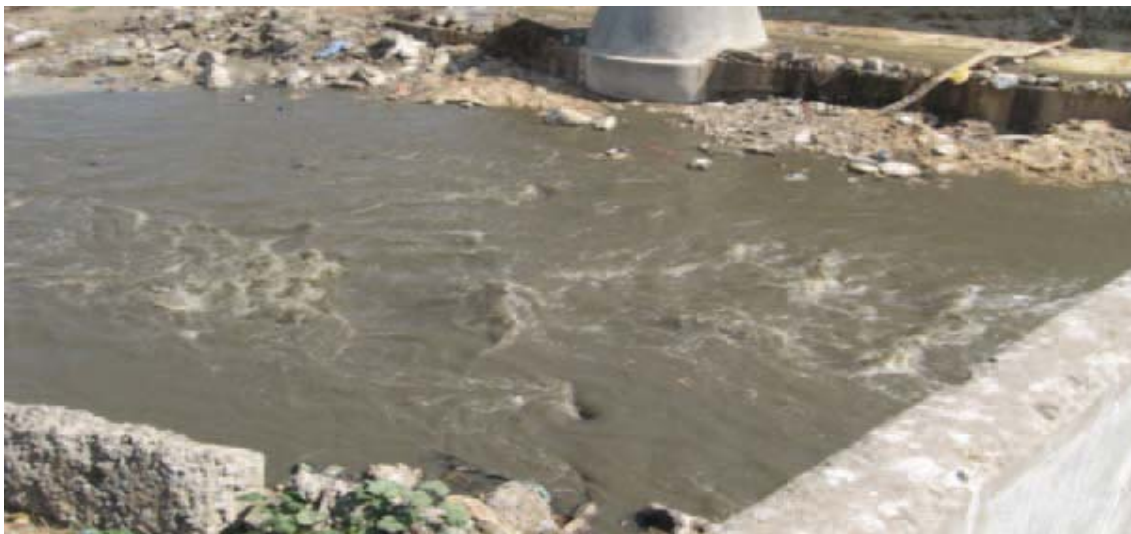
Blocked I&D at Murinala in Hyderabad
