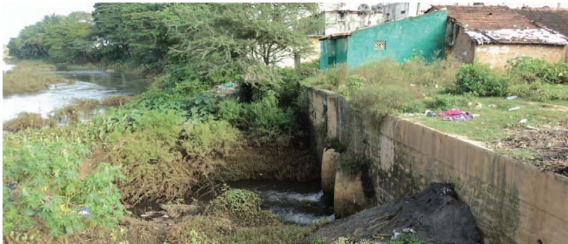
Flow of untreated sewage into River Bhadra in Bhadravati
