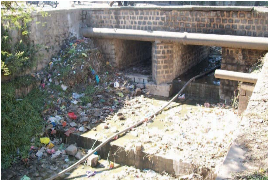
Sewage overflowing (after interception) and discharging directly into river Kshipra
