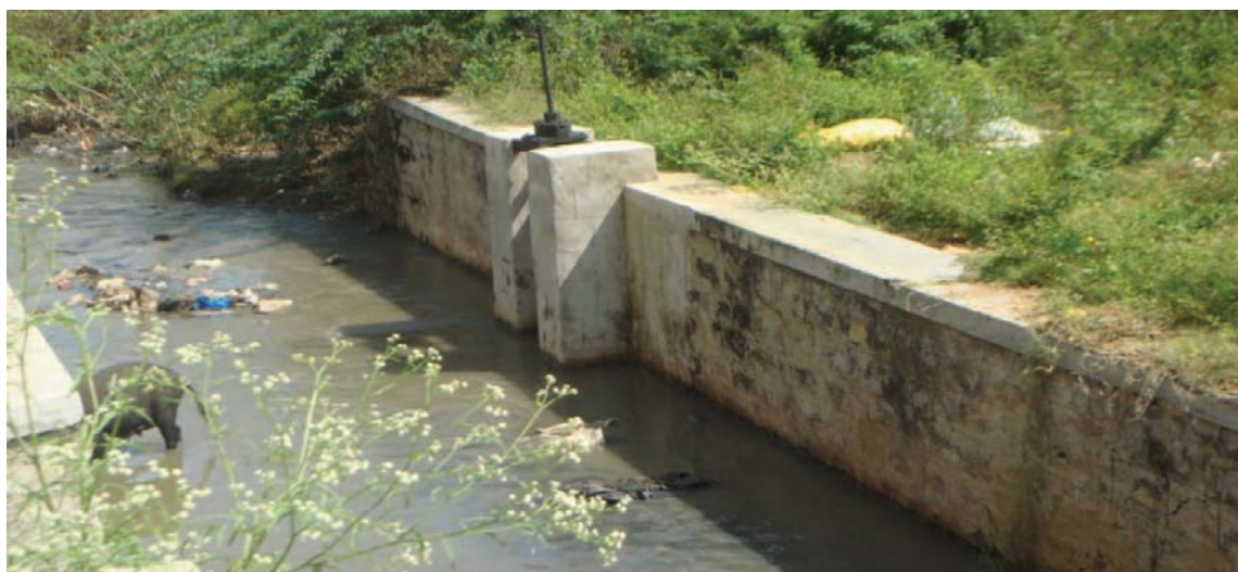
Blocked I&D at Davanagere
