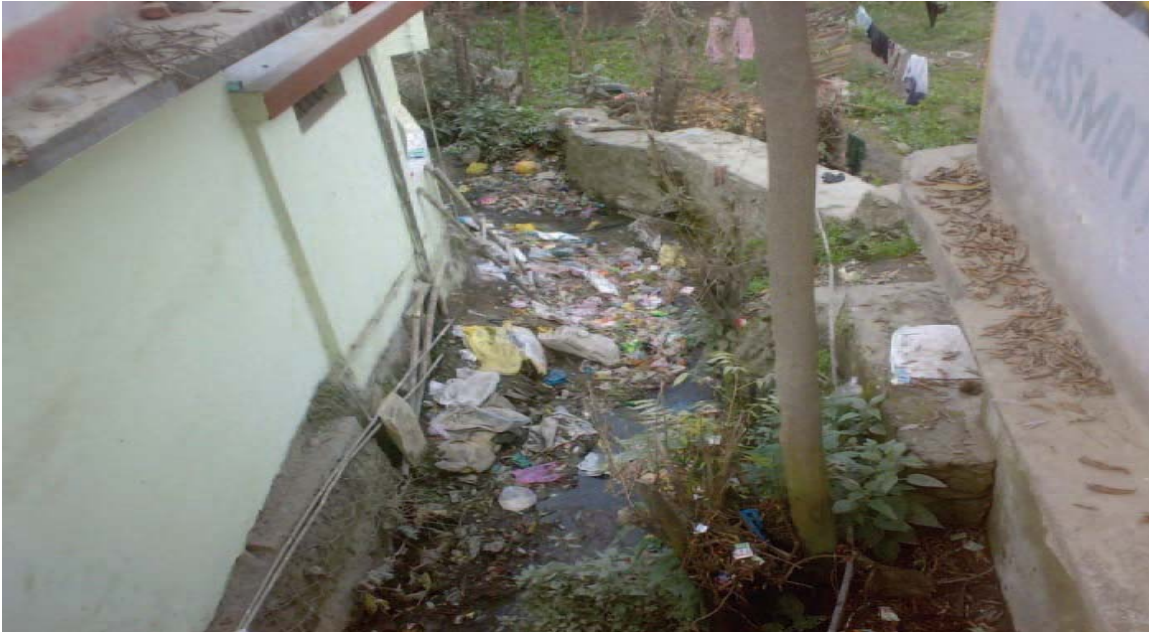
Untrapped drain in Srinagar
