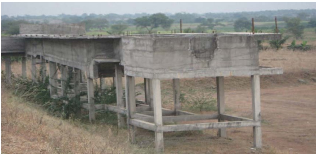
Abandoned works in Sangli
