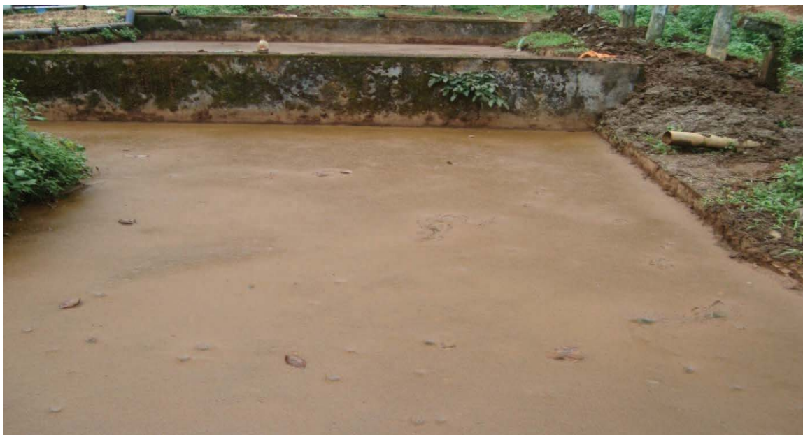
Sewage storage tank at Cheriyanavattom which over flows and sewage reaches the Njunangar stream
