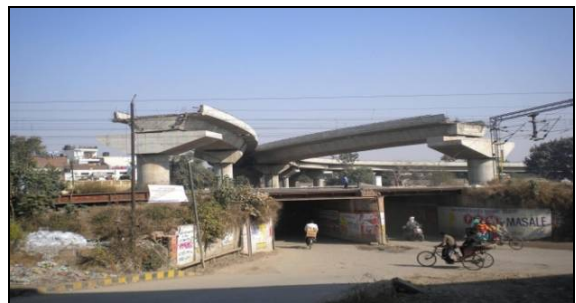
Damoria Bridge, Jalandhar (NR) – Sanctioned in 1997-98, approach portion completed, bridge portion not taken up.
