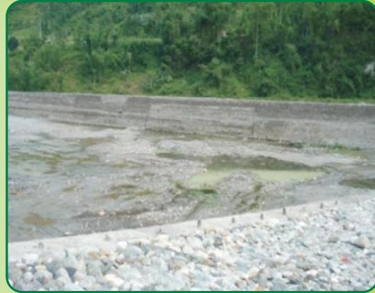
Incomplete work of Solid Waste Management at Shipchu (work was started four years back)
