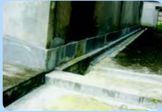
Tilting of building structure
