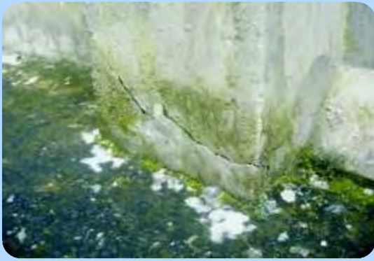
Cracks in RCC structure
