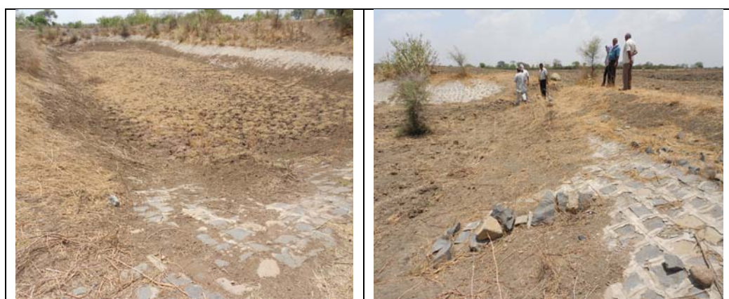
Photographs showing defective and mud filled water sources with broken sides - Jhalawar
