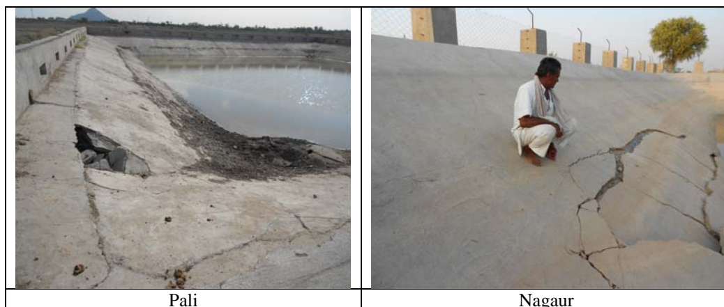
Photographs showing defective water sources with leakage/cracks (Pali and Nagaur)
